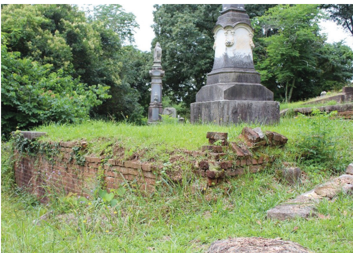
Before and after photos of the George W. Center lot demonstrate recent restoration results, with unsafe steps and a crumbling wall repaired.
